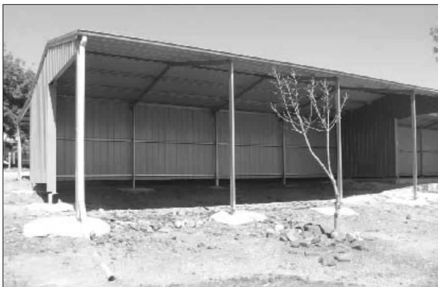
More work needed on Redesdale pavilion
